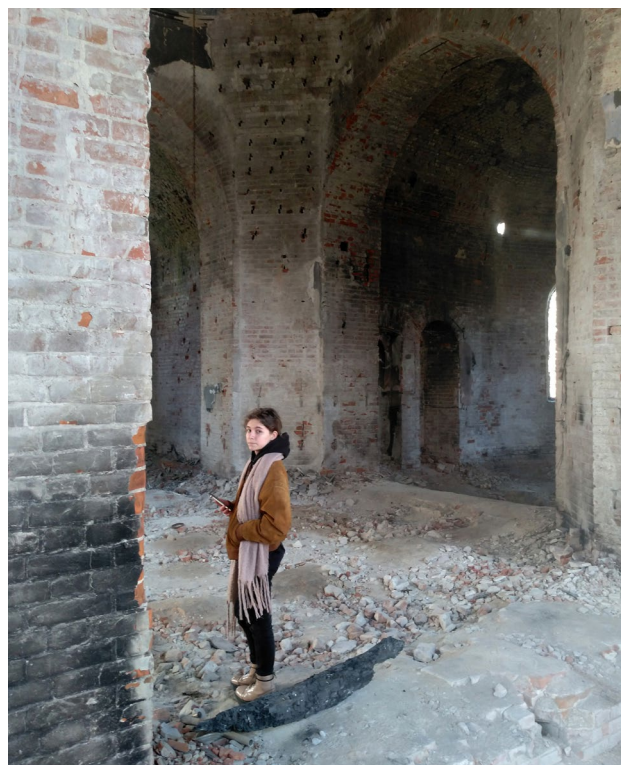
Fig. 10. Lukashivka village, Chernihiv Region, 2025. Recording damage in the early 20th-century Ascension Church.
